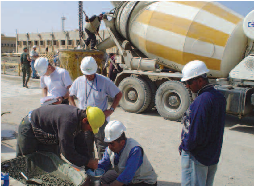
Perini and U.S. Army Corps of Engineers personnel test the concrete for use in building a new turbine generator at Nasiriyah Power Plant.
